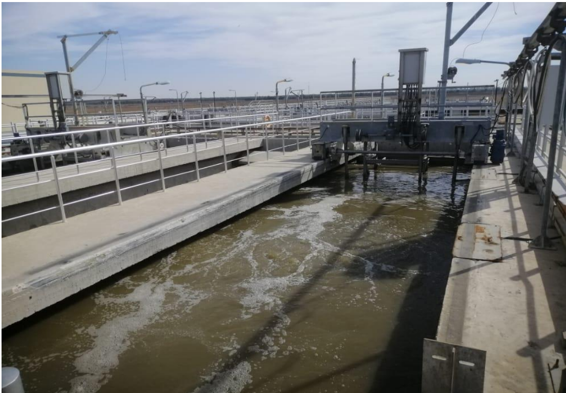
The Pre-Treatment Building Under Operation up to December 2021
