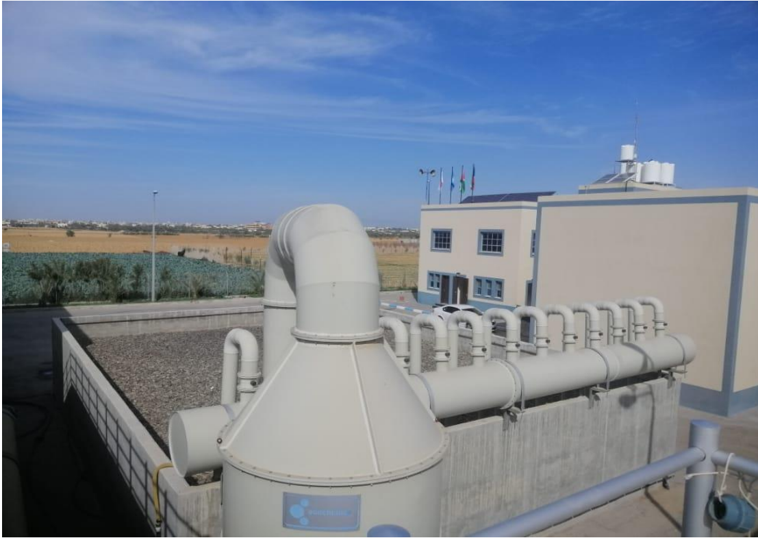
Bio-filter for Odour Treatment Under Operation up to December 2021
