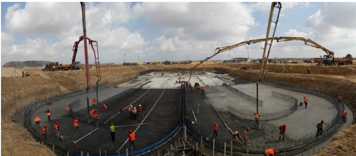
Casting Reinforced Concrete for the Foundation of the Aeration Tank on 20 June 2017
