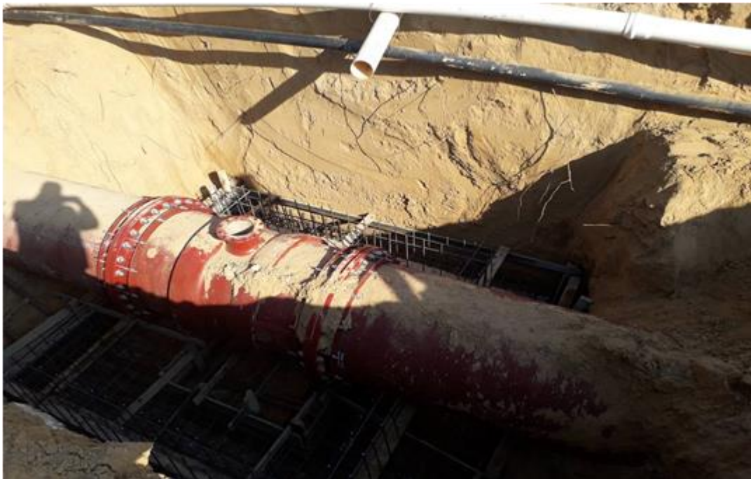
Ductile Iron Pipes Entered Gaza and Installed on Site for the Effluent Pressure Lines (CMWU Package) up to Completion in June 2020
