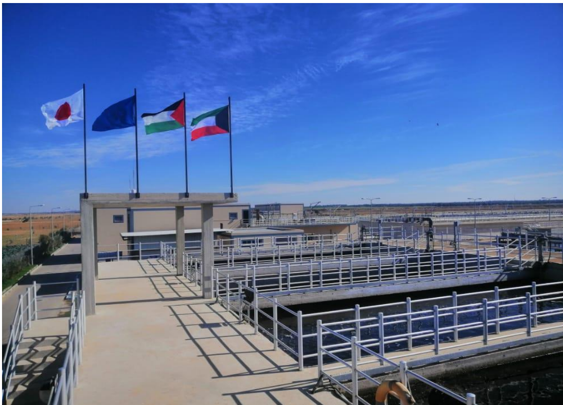
Sand Filter Under Operation up to December 2021
