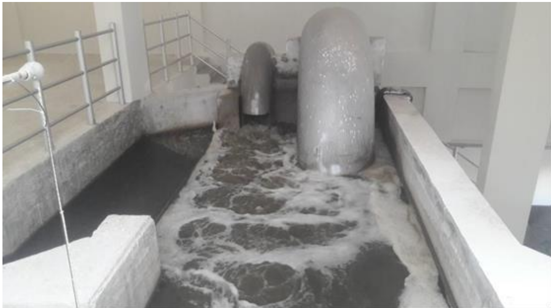
Wastewater Introduced to the Plant from the Inlet Pipe at the Pre-Treatment Building on 09 September 2019
