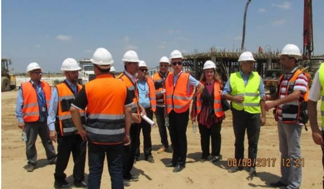
Site Visit of H.E. Mr. Takeshi OKUBO; the Ambassador of the Palestinian Affairs and the Representative of Japan to the Palestinian Authority, to KY WWTP on 08 August 2017
