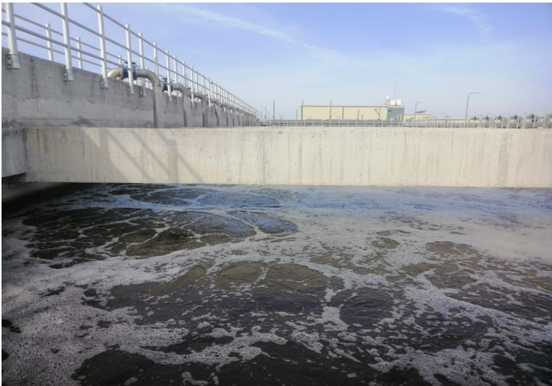
The Aeration Tank Under Operation up to December 2021
